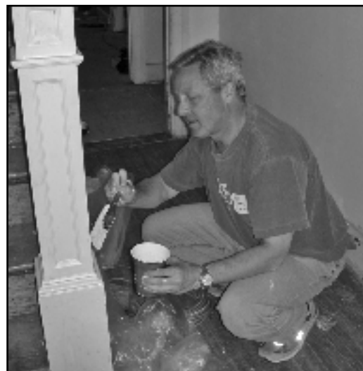
Albert (Sonny) Small, Jr., 2008 Yachad Bash honoree, paints a staircase at the Sukkot in Spring house renovated by the Real Estate Affinity Group.
