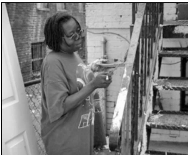
Homeowner Sheila Brown works with the Mitzvah Project crew to repair her house on Father's Day.
